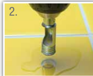
2. Continue drilling and raise the bit to 90 degrees to complete the hole in the tile.
